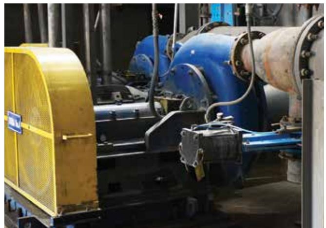
The pump (pictured), cyclones and mill work together to determine circuit classification system efficiency.
